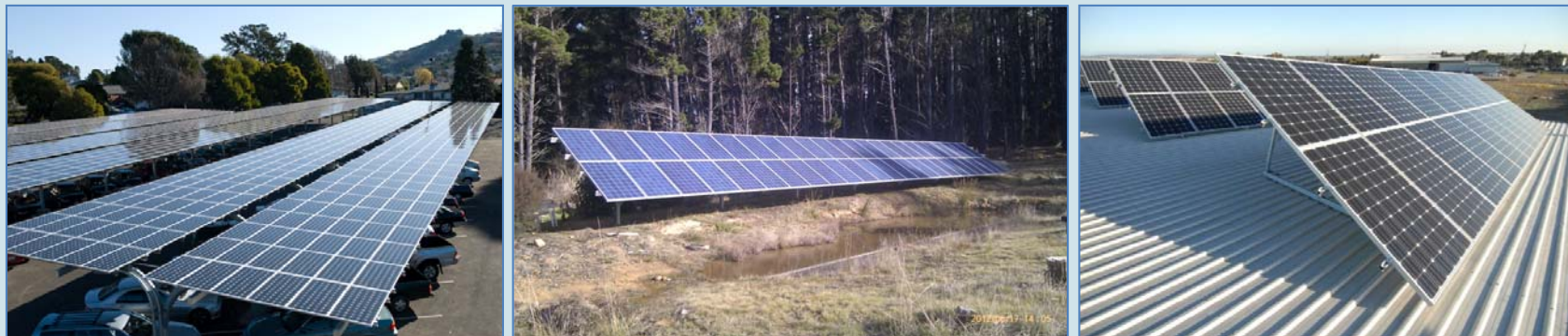
Figure 3: Solar Panels as Car park shading, ground and roof mounted.
