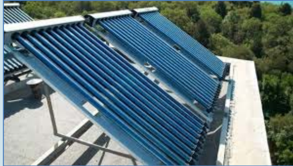
Figure 6: Roof Mounted Solar Hot Water System
